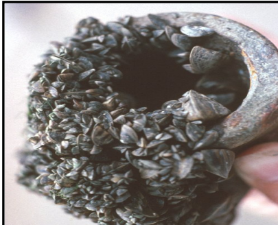
Zebra mussels encrusting pipe orifice.
